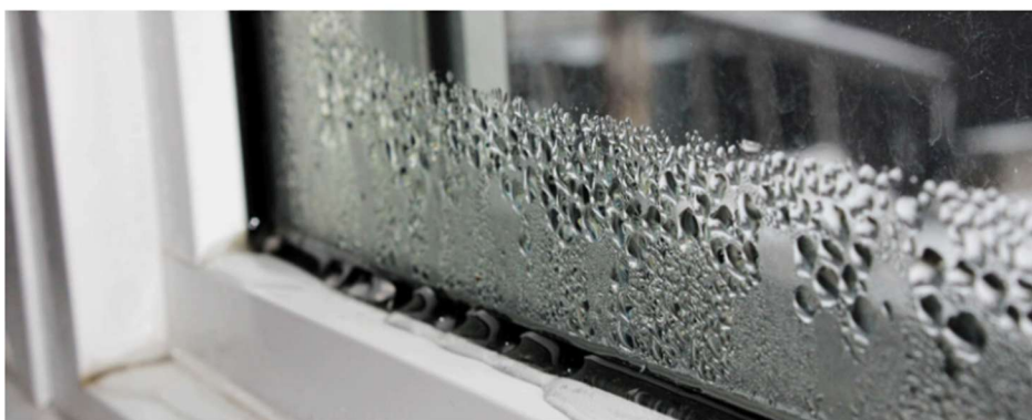
Image 1. Picture showing the condensation phenomenon inside the sealed units
