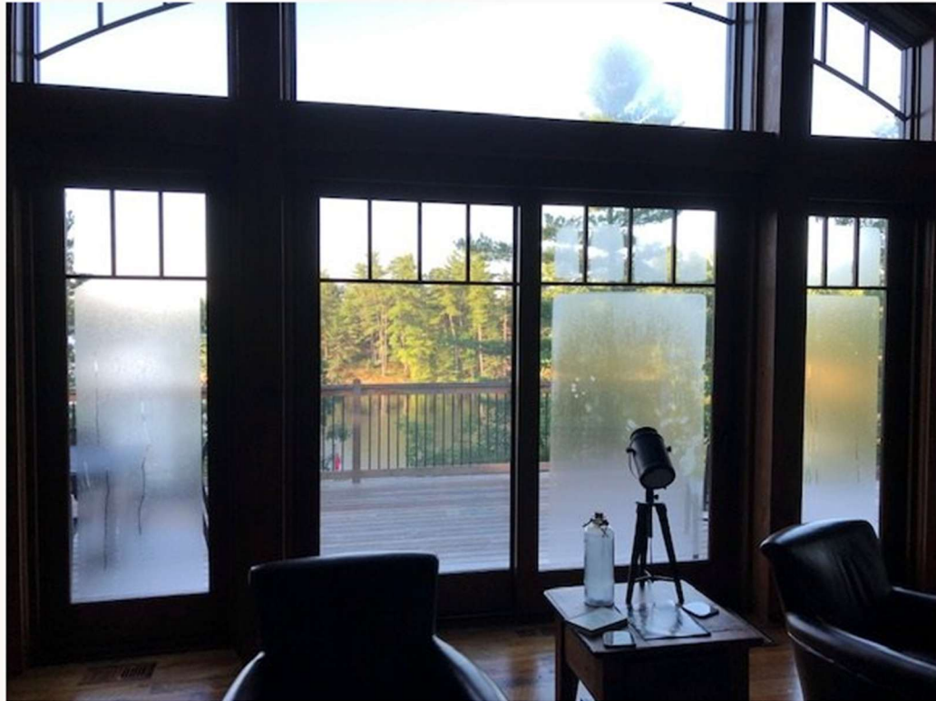
Image 2. Picture showing the condensation phenomenon outside the sealed units
